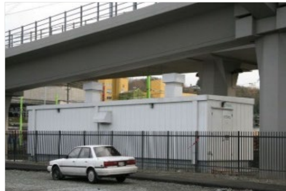
Figure 2-6. Typical Traction Power Substation
