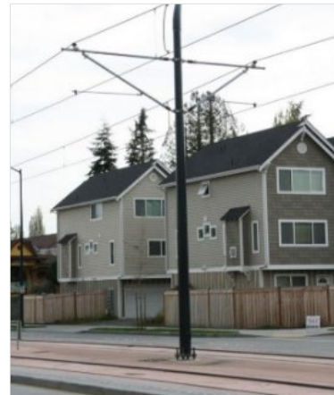
Figure 2-5. Typical Overhead Catenary System
