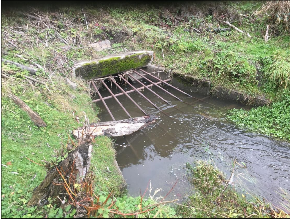
Figure N4.D-24. Longfellow Creek Culvert – Southwest Genesee Street Culvert inlet on the golf course, taken October 10, 2019.
