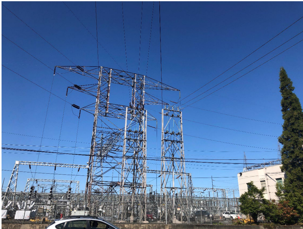
Figure N.5B-DUW-48. #5139b, Seattle City Light South Receiving Substation Switchyard, 3839 4th Avenue South (WISAARD #725921)
