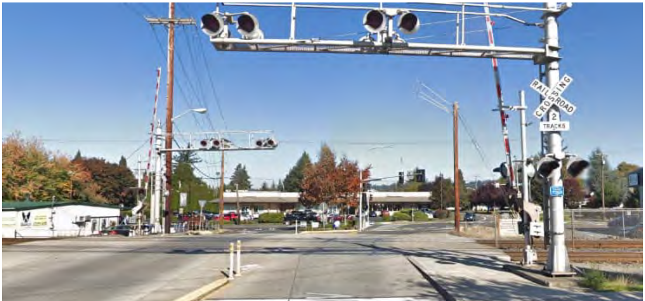
Figure 120-3: Two-Quadrant Vehicular Automatic Gates with Flashing Lights
