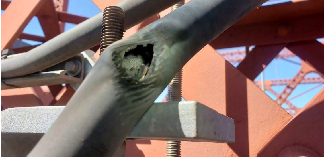
Figure 6. Melted power cables for Portland Streetcar during the June 2021 Heat Dome Event
