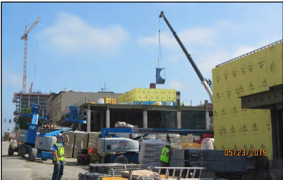
N140 - Crews Lowering Coupler for Ventilation Fan to Noise Attenuator at North Headhouse.
