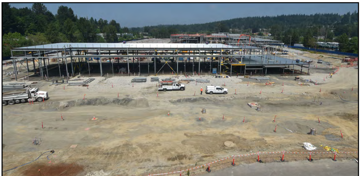
OMF East looking north taking shape with yard scope and steel structure framing on May 31, 2019
