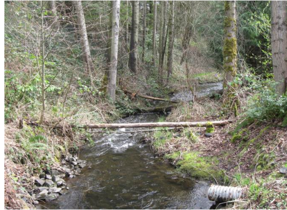
McAleer Creek near the outlet of the culvert under I-5, looking downstream (culvert at right is not the I-5 culvert)
