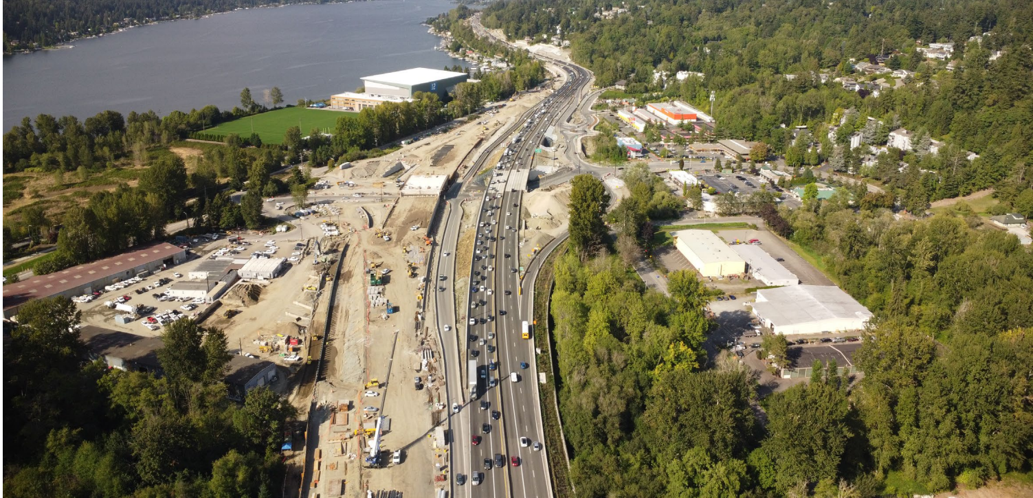
S1: NE 44th Interchange & BRT station looking north (September 2024). Southbound roadway taking shape (center). BRT station to be located between NB and SB I-405.
