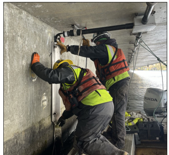
Crews removing anchor cable guard on floating bridge while investigating cathodic protection components
