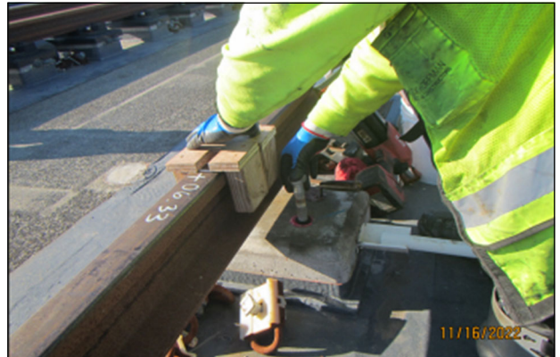
E130 Seattle to South Bellevue: Installing new nylon inserts on floating bridge, westbound
