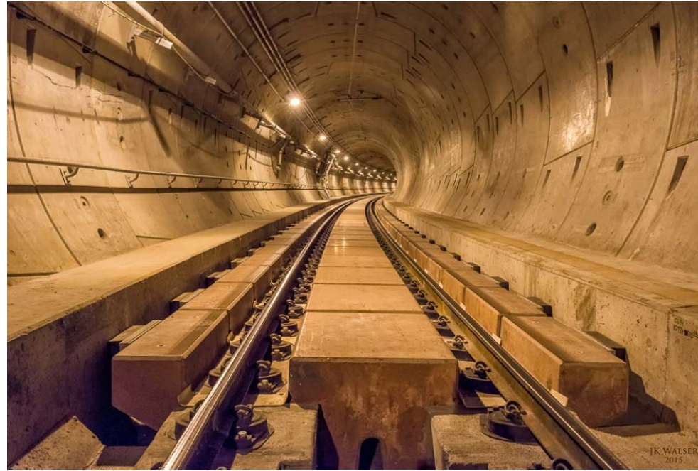
Floating Slab under UW Campus to mitigate noise and vibration
